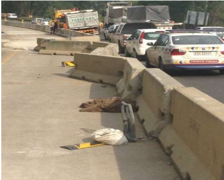
Figure 33: Incorrect Use of Barriers in the Work Zone
