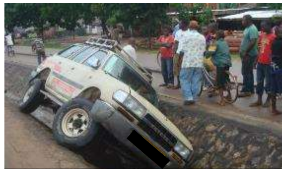
Dangerous deep open drain parallel to road
