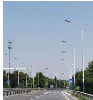
Protected Street Lights
