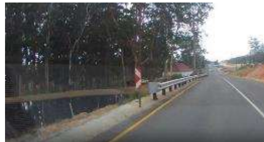
Barrier too short, bull nose unacceptable
